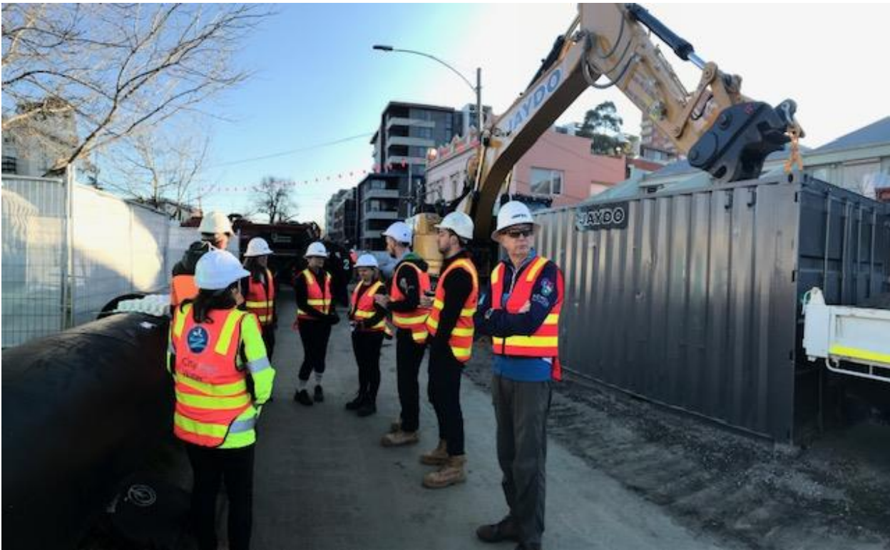
Photo 4: CRG Group discussing construction methodology with Dwayne Deprez (CWW Project Manager), Daniel Schaede (Jaydo Project Engineer) and Ray Coffey (Project Foreman).
