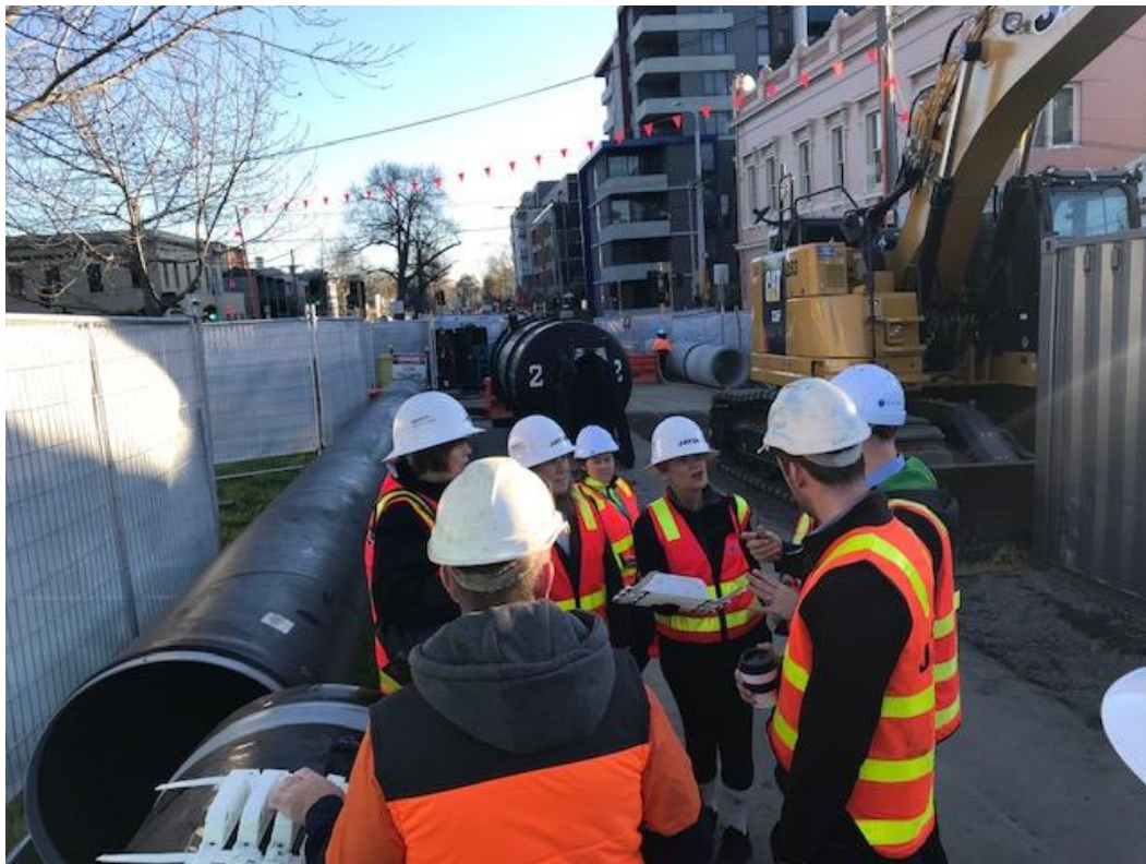
Photo 2: CRG group discussing pipe fitting methodology and fabrications with Dwayne Deprez (CWW Project Manager), Daniel Schaede (Jaydo Project Engineer) and Ray Coffey (Project Foreman).
