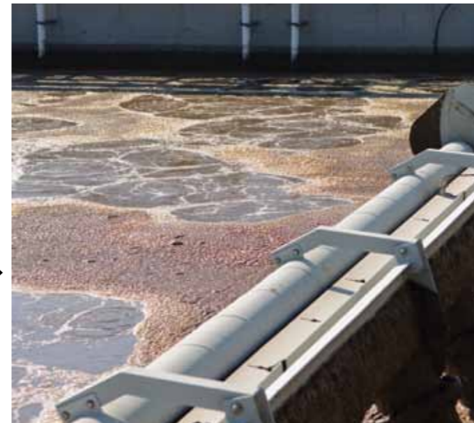
Biosolids are separated from the treated sewage.
