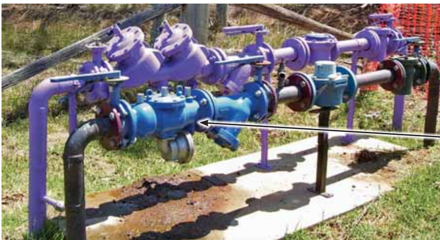
Example 1: High Risk Reduced Pressure Zone Device
