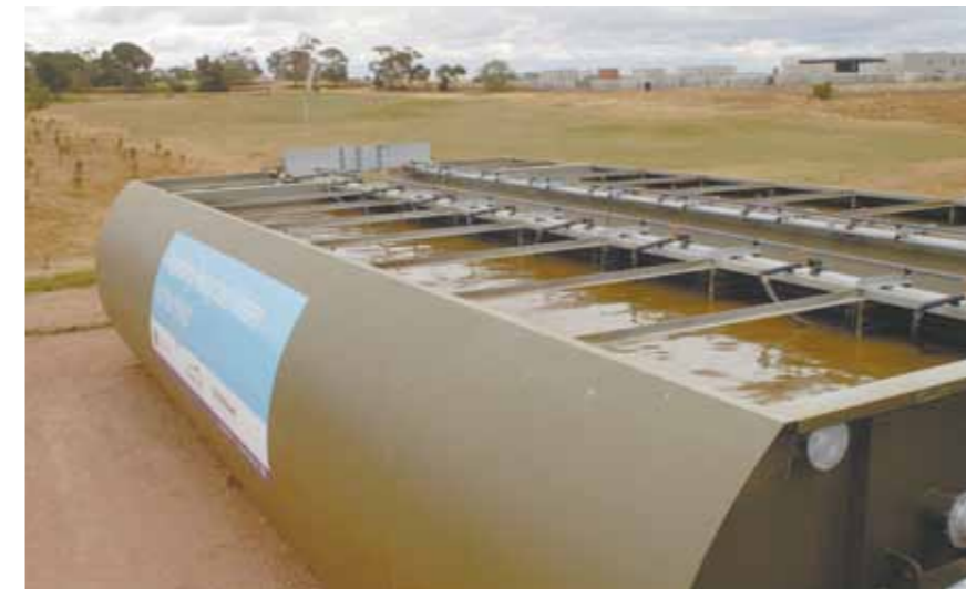
The Sunshine Golf Course Recycled Water Sewer Mining Project
